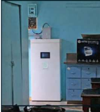
A Sonnen energy-storage system powers S.U. Matruillas, a school for grades K through 9 serving more than 150 students in the remote town of Orocovis, Puerto Rico.
